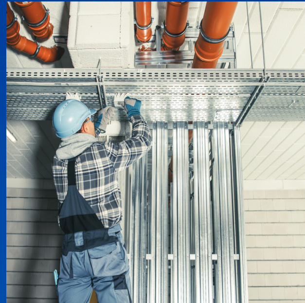
Electrical Infrastructure and Pre-fabrication Services
